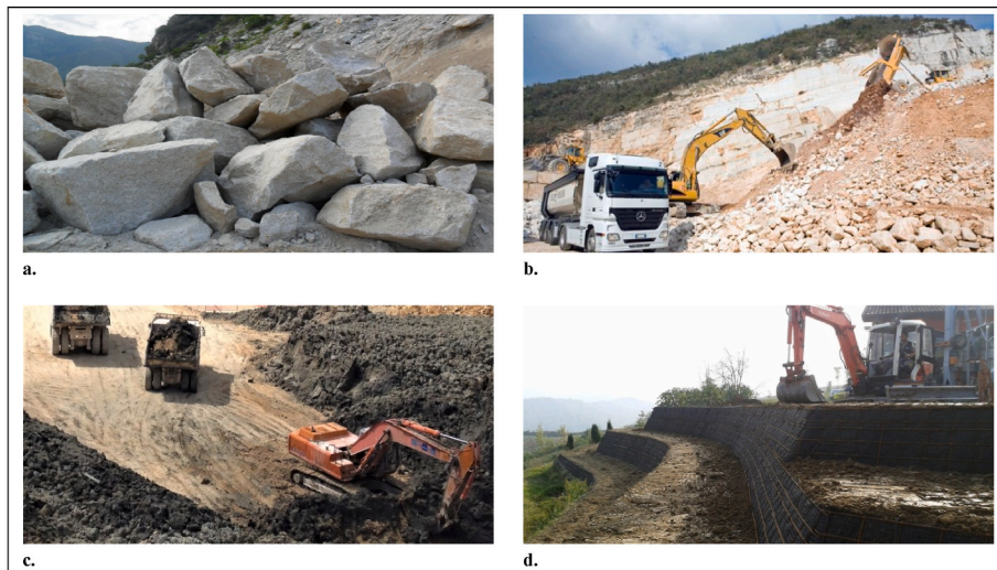
Fig. 2. a. Quarry boulders; b. Arid quarry mix (Tout Venant); c. Receiving excavated soil and rocks; d. Reuse of excavated soil and rocks in artificial embankment.
