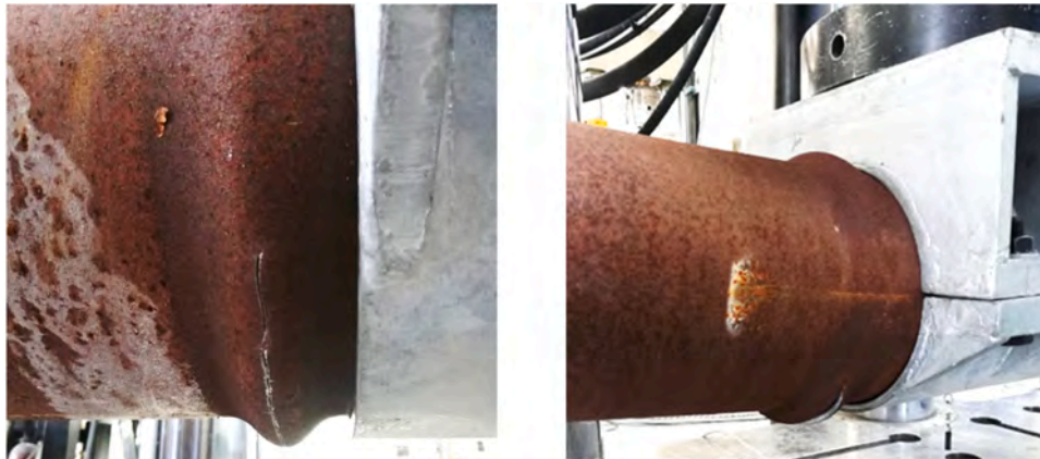
Fig. 11. Bulges and cracks near the rigid stub.
