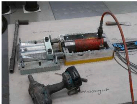
(b) Attaching the strip, fixing the frame, and prestressing it up to desired pre-strain level
