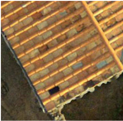
(c) Broken Tile
