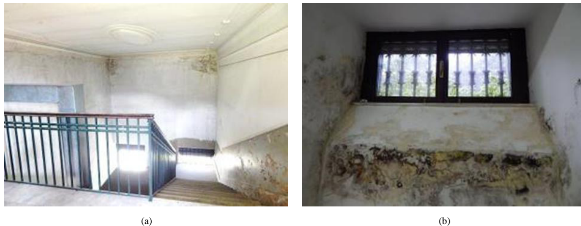
Fig. 8. (a) Infiltration due to the rainwater to the roof slab; (b) Infiltration due to rainwater rebound, with mold and condensation. Wall basement, Northern prospect.
