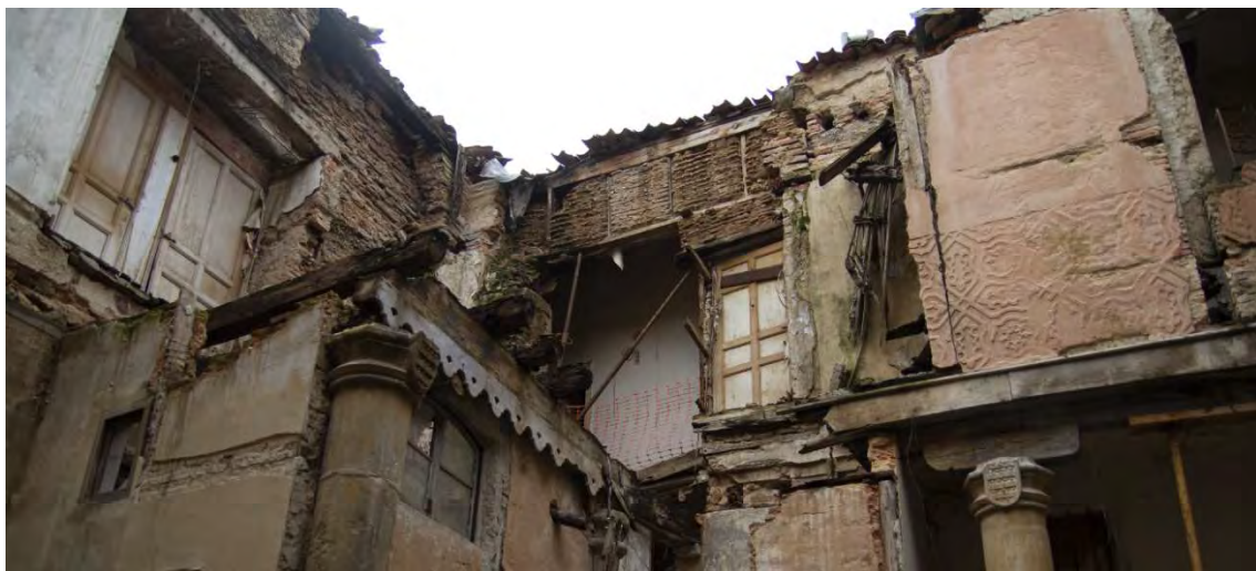
Figure 8. Main cloister; detail of a collapsed wooden floor due to the rotting of the beams.
