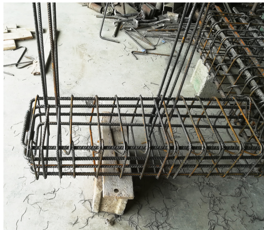
FIGURE 2.24: Joist reinforcement warping the longitudinal beam rebars.
