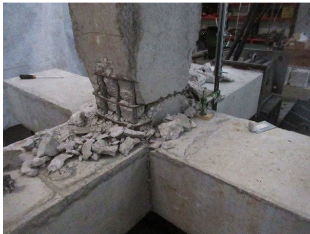
FIGURE 4.16: Final damage in the beam of J_01 – C specimen.
