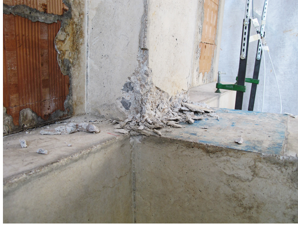
FIGURE 4.50: Final damage in the beam of J_{01\_S} - M^- specimen.
