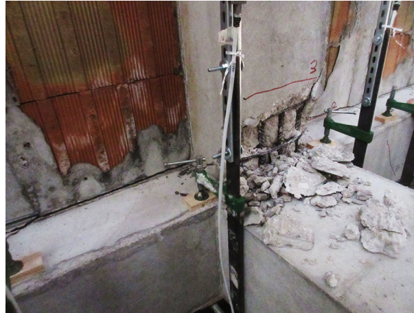
FIGURE 4.45: Final damage in the beam of J_{01\_S} - C specimen.
