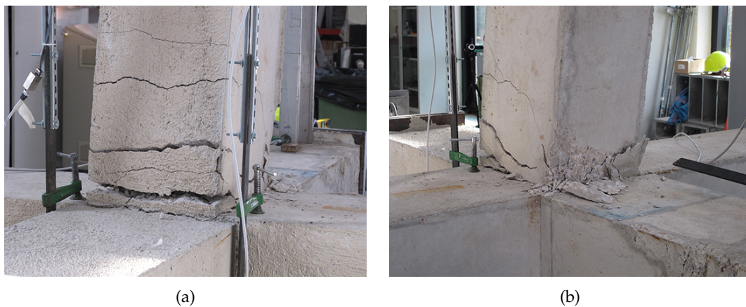
FIGURE 4.18: Final damage on beam tension (a) and compression (b) sides of J_{01} - M^+ specimen.
