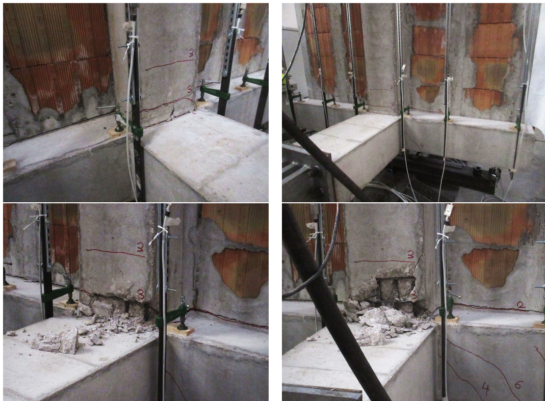
FIGURE 4.42: Crack pattern evolution on the joists side of J_{01\_S} – C specimen.
