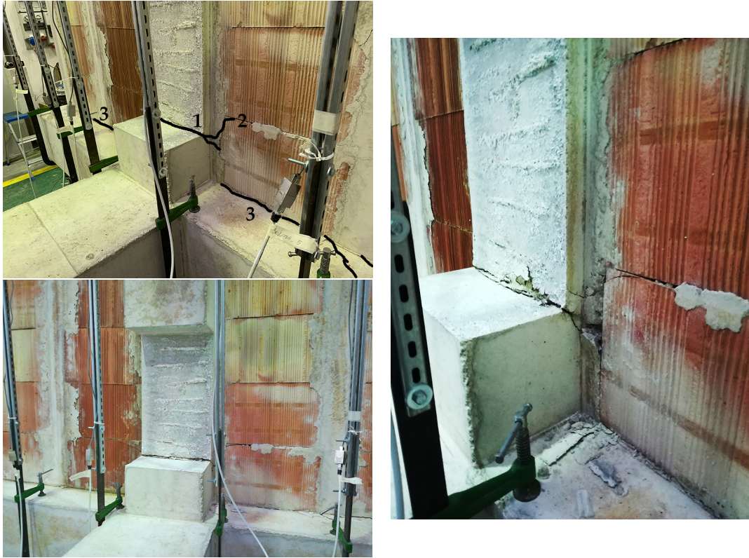
FIGURE 4.88: Crack pattern evolution on the joists side of J_{02\_S} - C specimen.
