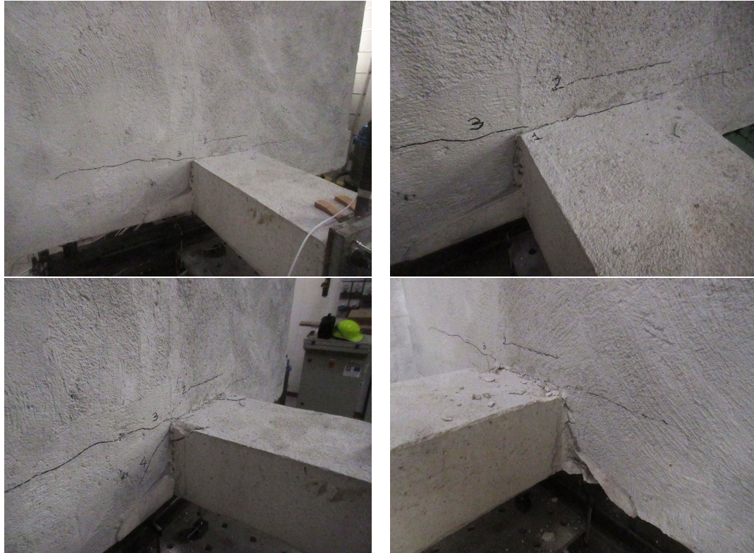
FIGURE 4.43: Crack pattern evolution on the slab side of J_{01\_S} - C specimen.
