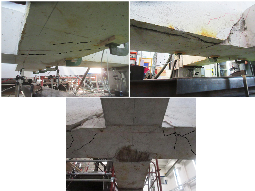
FIGURE 4.40: Crack pattern evolution in the joint and longitudinal beams of J_{01\_S} – Geolite – C specimen.
