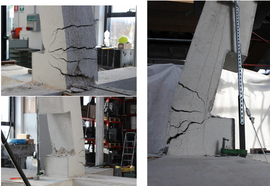
FIGURE 4.73: Final damage in the beam of J_{02} - M^- specimen.
