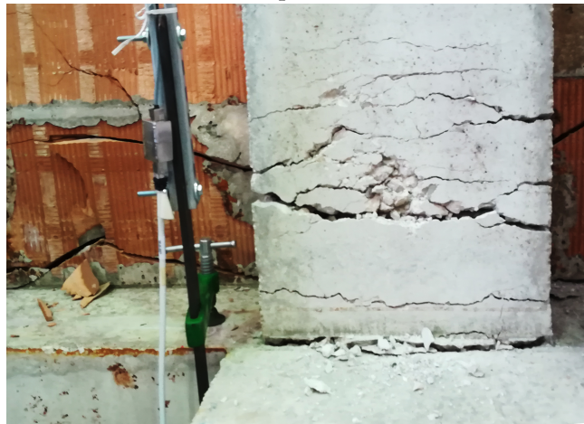
FIGURE 4.49: Final damage in the beam of J_{01\_S} - M^+ specimen.
